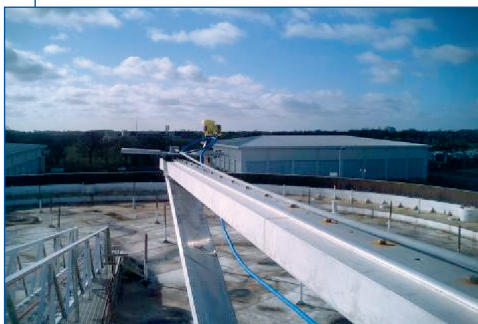
Radar level measurement as part of an overfill protection system
